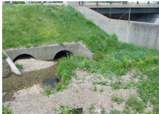
These culverts have filled in with sediment and require maintenance. Improvements to increase the detention area upgradient could easily be made; however, periodic maintenance is crucial to the performance of the BMP.
