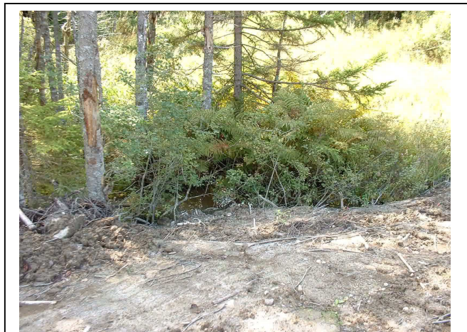
The upgradient area of this wetland was not properly stabilized and maintained, causing large amounts of sediment to deposit in the wetland. The cost to retrofit this stormwater structure will be more costly than if the original specified construction and maintenance plan had been followed.
