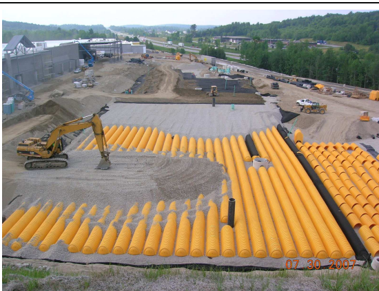
Subsurface detention and infiltration galleries under a parking lot save space. With visible and adequate pretreatment and frequent maintenance, they can work well and will help recharge groundwater. Without pretreatment and maintenance, they quickly fill with sediment and may fail.
